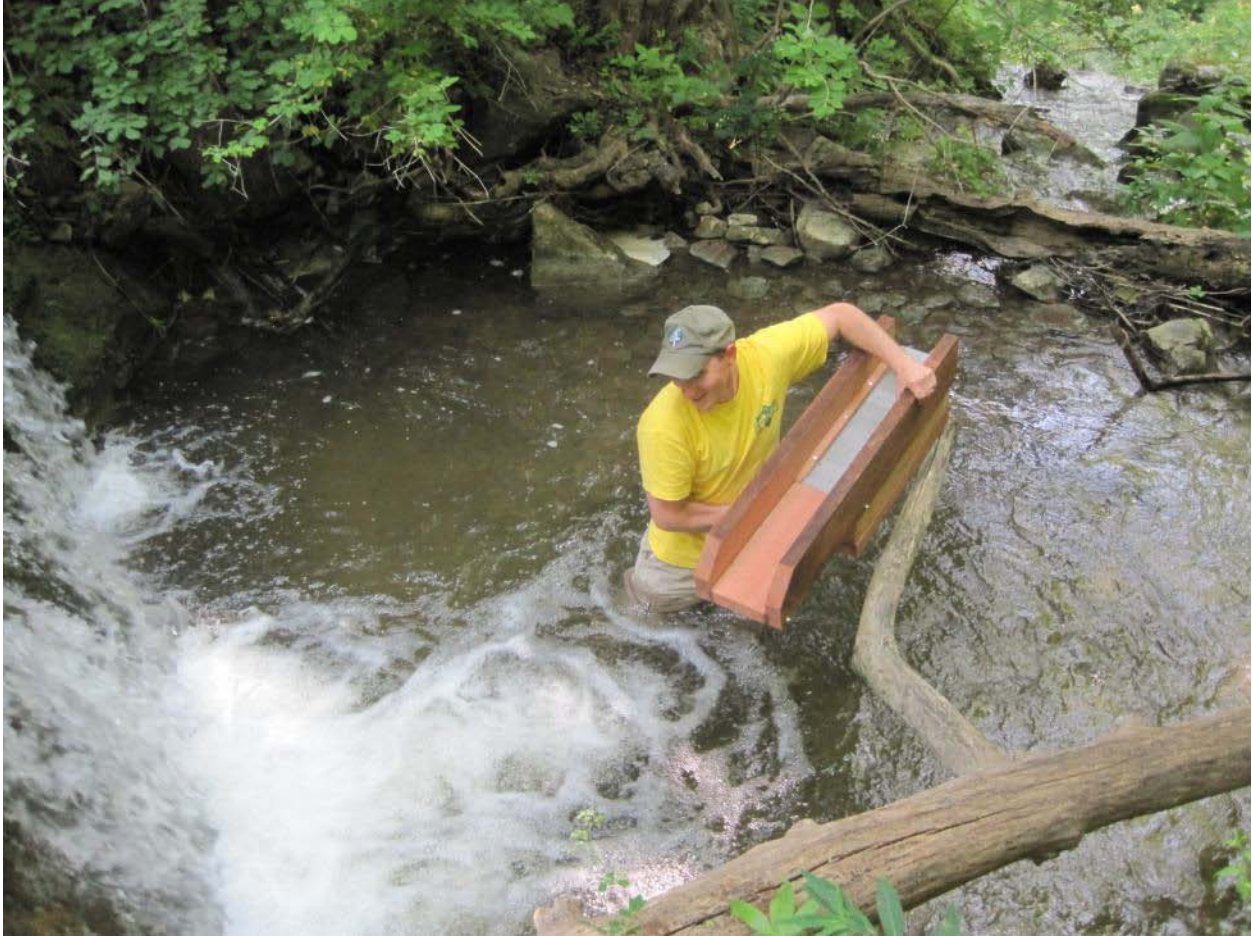
Identifying a suitable intake location for our off-grid bathhouse at Oxbow Falls County Park.
