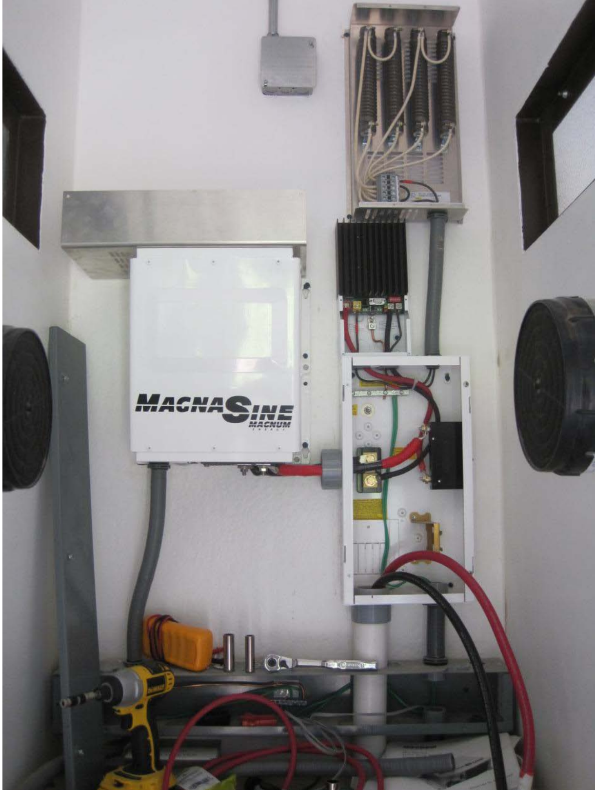
Partially through the installation of the battery bank, inverter, charge controller, and diversion load.
