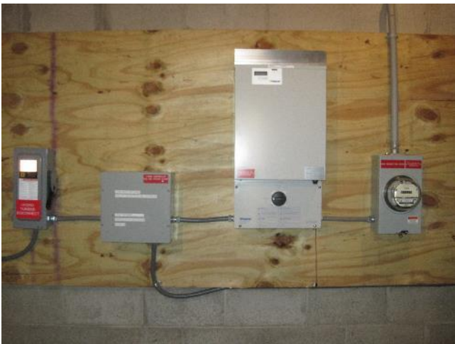
Disconnect, controller, inverter, and energy meter
