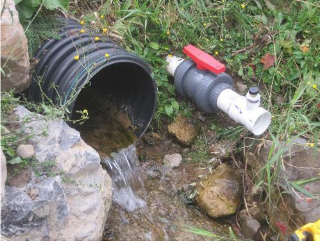
Ball valve and vacuum relief valve at intake
