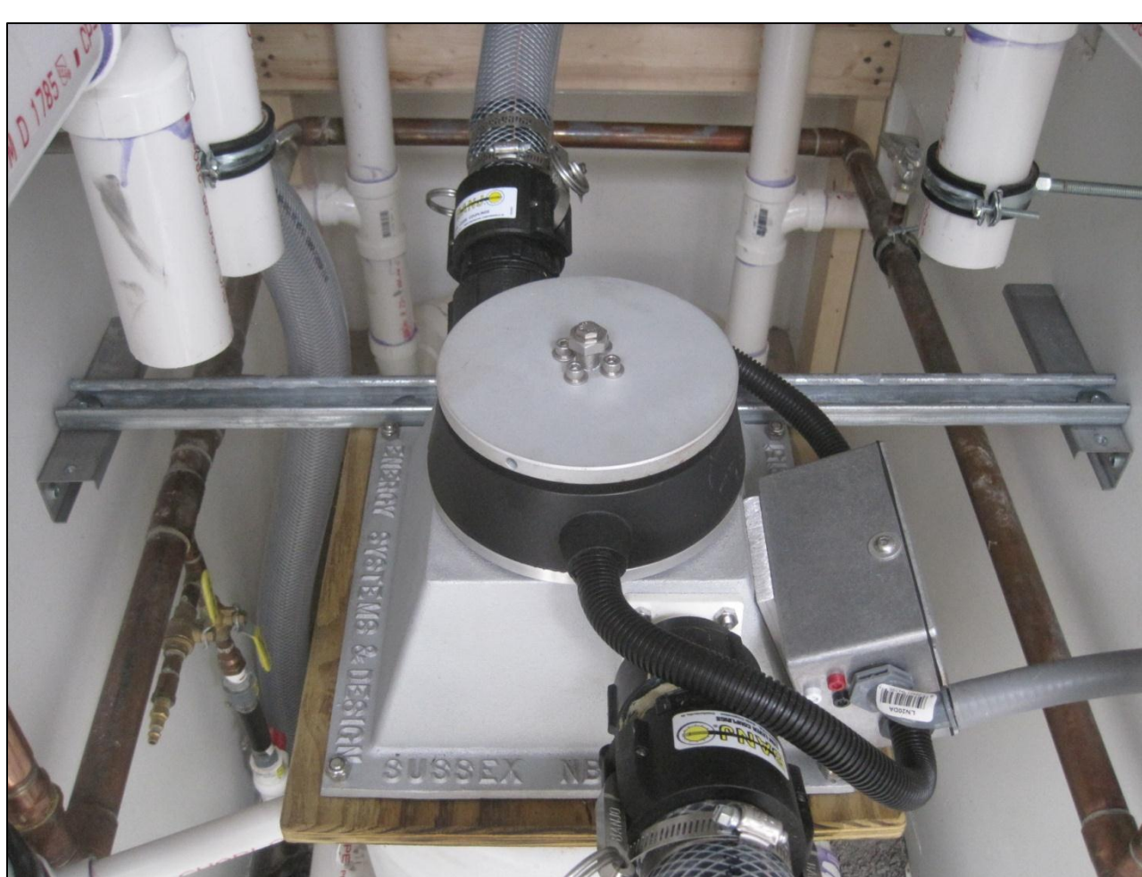
The turbine is operating at 325 Watts (3,100 kWh/year) and supplies 48 VDC.
