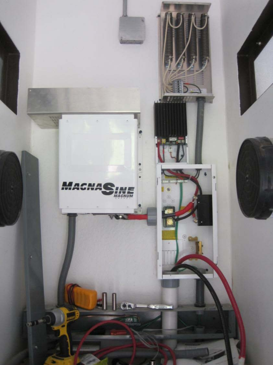
Wiring an off-grid micro hydro system
