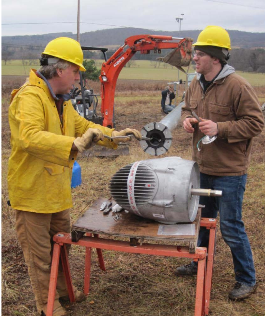
Wiring the alternator
