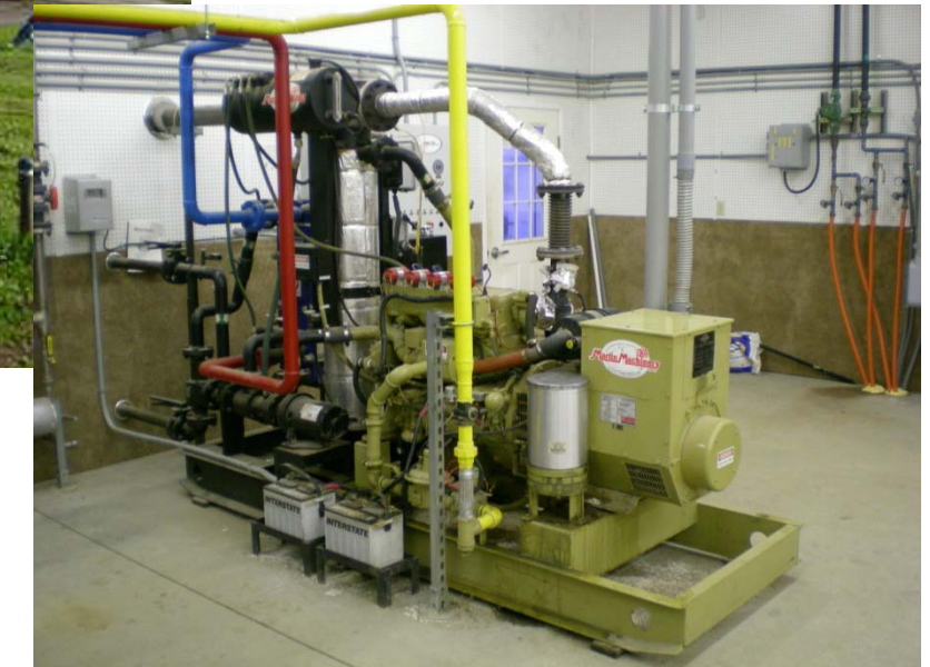
50kW ICE/electrical generator
